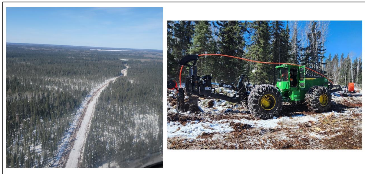
Figure 4 New access corridor and buried fibre optic cable installation on TPK claims, March 2026.
